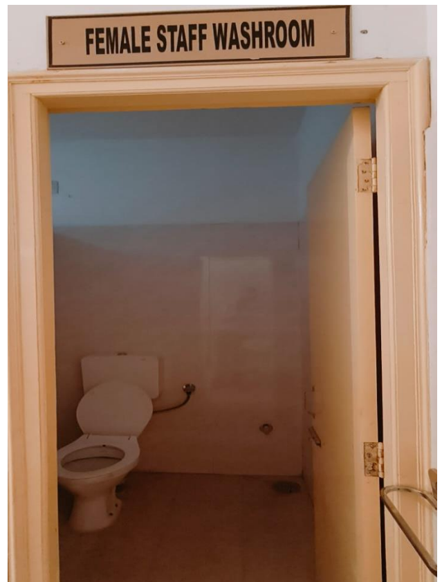
Upper Floor Toilet for Female Staff
