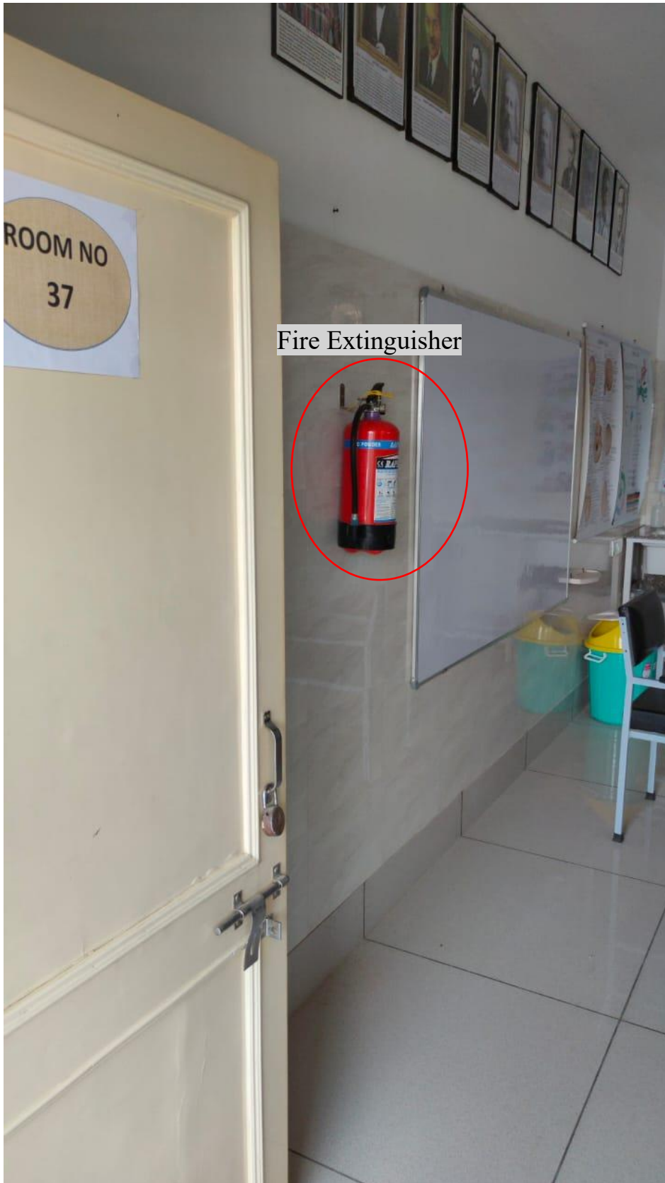
Science Lab Fire Extinguisher
