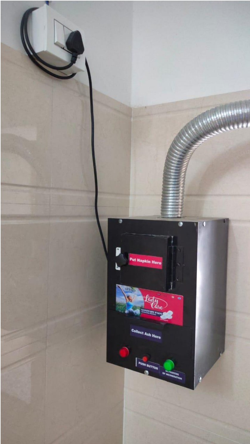
Incinerator in Upper Primary Girl's Toilet
